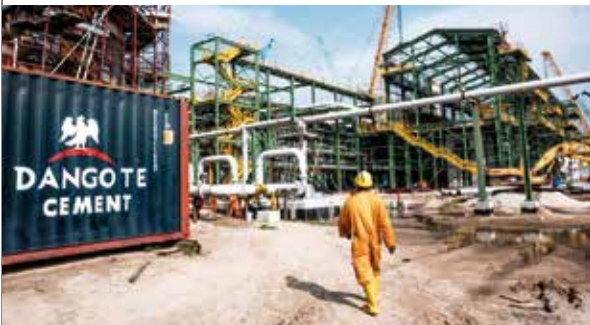
Left: Work proceeds on the construction of the Dangote Refinery. When complete it is expected to double Nigeria's oil refining capacity.
